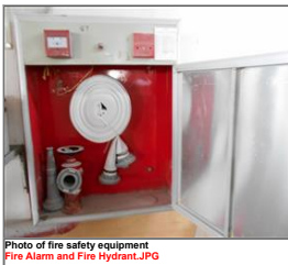
Photo of fire safety equipment Fire Alarm and Fire Hydrant.JPG
