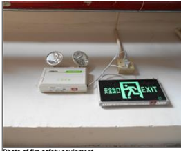
Photo of fire safety equipment Emergency Lights and Exit Sign.JPG
