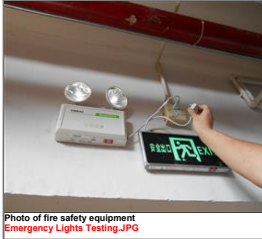
Photo of fire safety equipment Emergency Lights Testing.JPG
