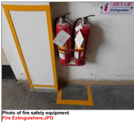
Photo of fire safety equipment Fire Extinguishers.JPG
